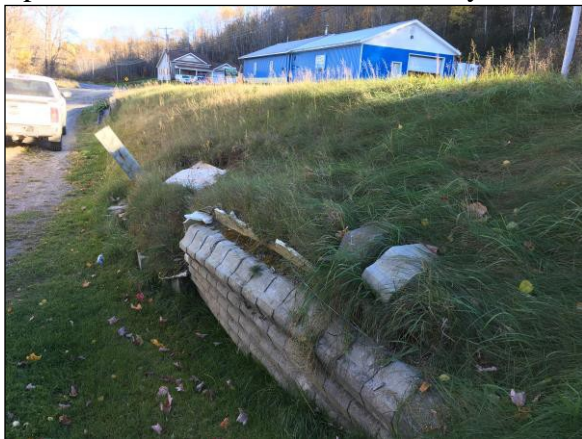
Figure 7 A section of retaining wall holding up an embankment below the road surface is compromised and threatening a private driveway below.
