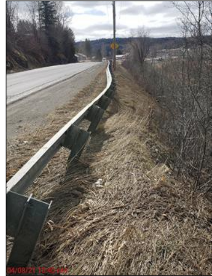
Figure 5 Compromised guardrail high above a steep slope along the road.
