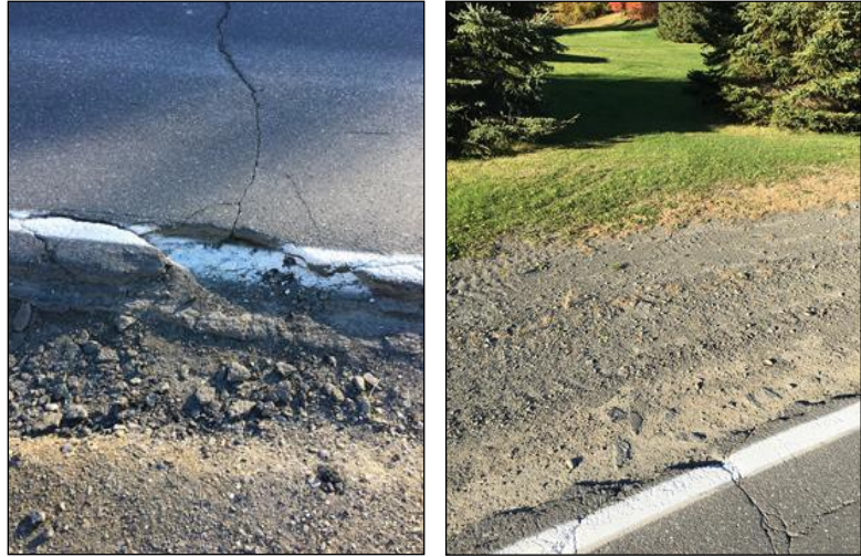
Figure 4 (left) Road surface cracking and breaking apart near edge, creating instability for vehicles, bicycles, and pedestrians using shoulder. (Right) Gravel shoulder compromised by erosion, wash boarding, and pavement cracking.
